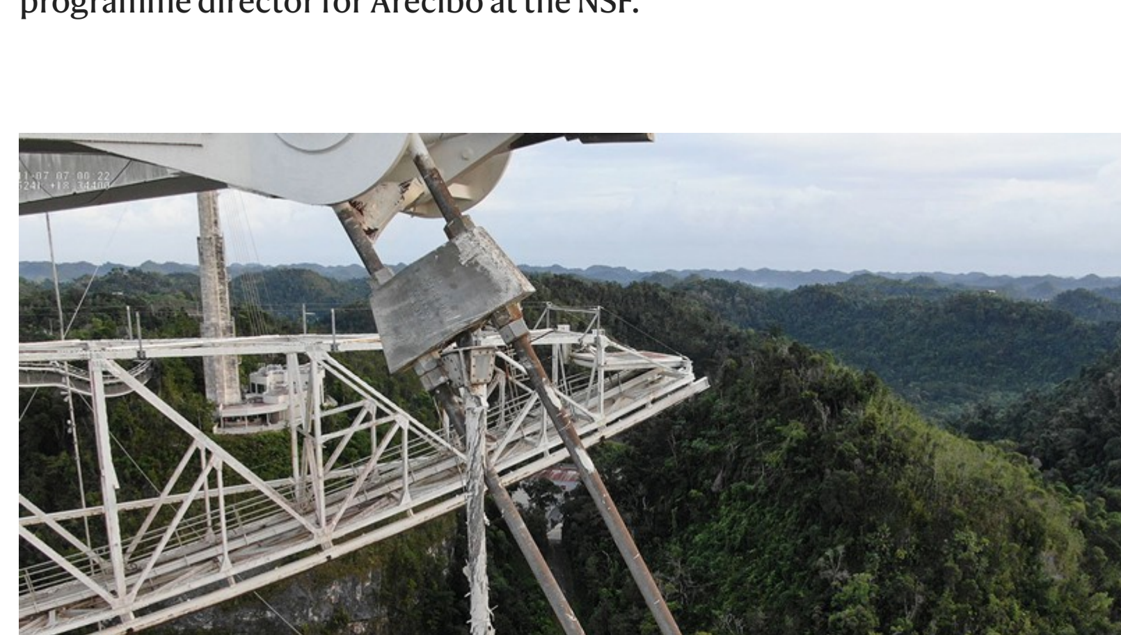
The main cable that failed experienced wire breaks (shown) before its sudden and unexpected collapse. Credit: University of Central Florida/Arecibo Observatory
