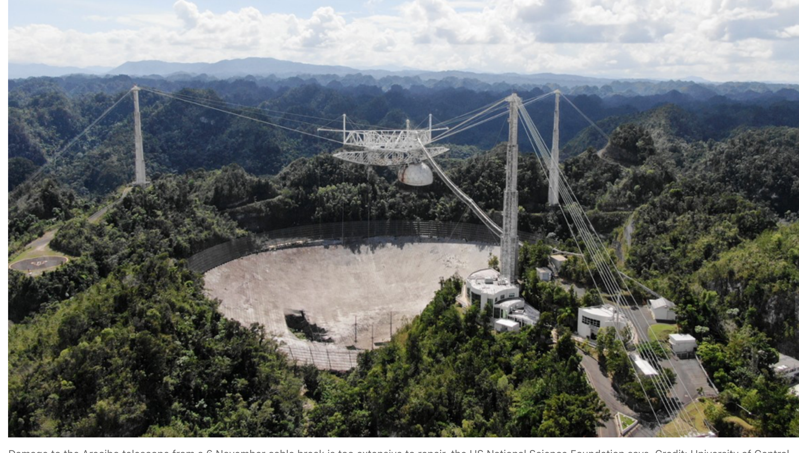
Damage to the Arecibo telescope from a 6 November cable break is too extensive to repair, the US National Science Foundation says. Credit: University of Central Florida/Arecibo Observatory
