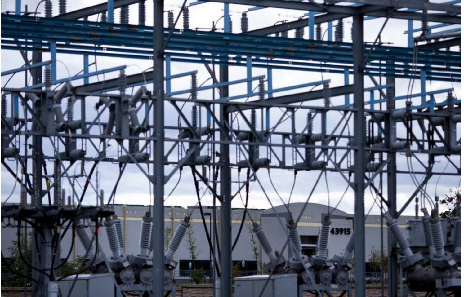
A data center in Ashburn, Va., seen past a Dominion Virginia Power substation serving it.
